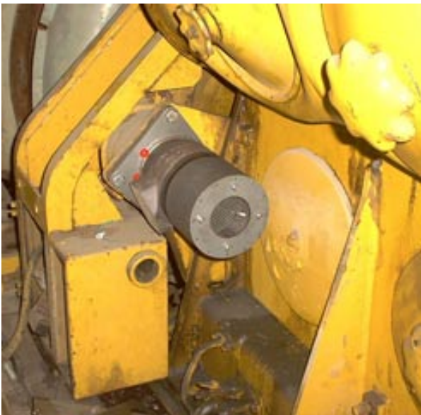
Pictured: ATS103-3636 on EMD 16-645 generator set
